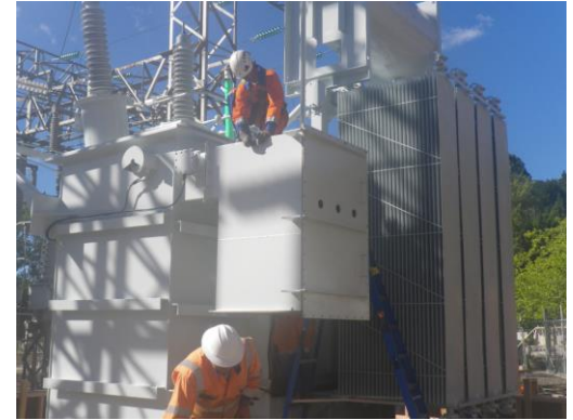
Installed in final location in switchyard
