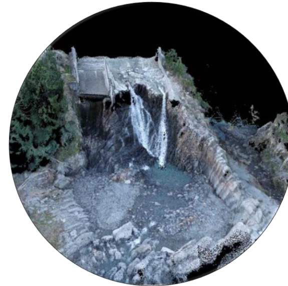
3D model of the Waihopai Spillway with a small flow over it, showing damage from the recent flood event. This model will be used to design the repairs.
