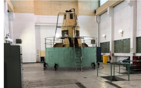
Existing Waipori 4 generator scheduled for replacement
