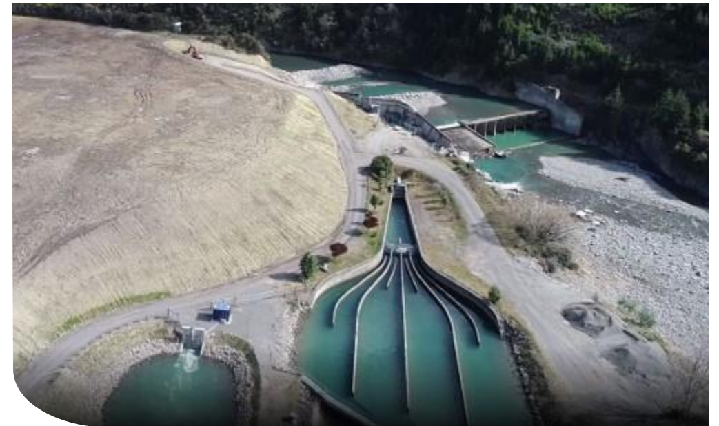
New Branch infiltration gallery with discharge into the Argyle Canal on the left
