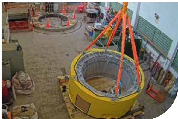
Unpacking new stator, the stationary part of a rotary system, at Waipori 4 station
